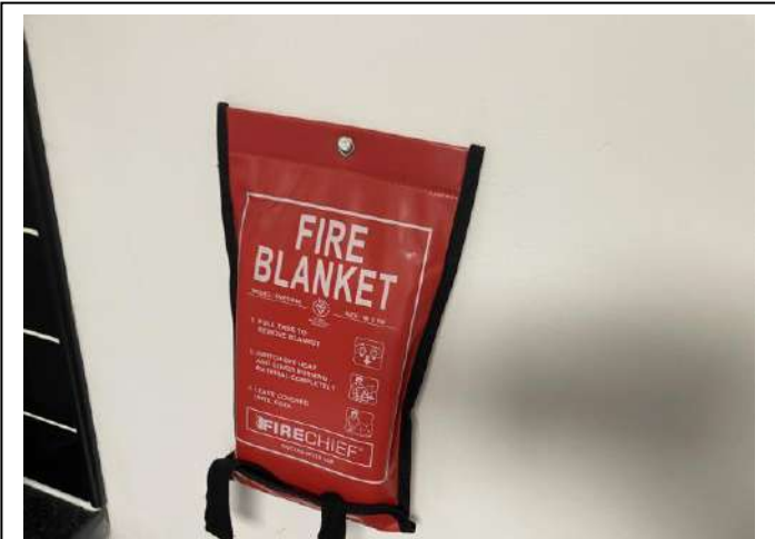
Location – Kitchen Wall
