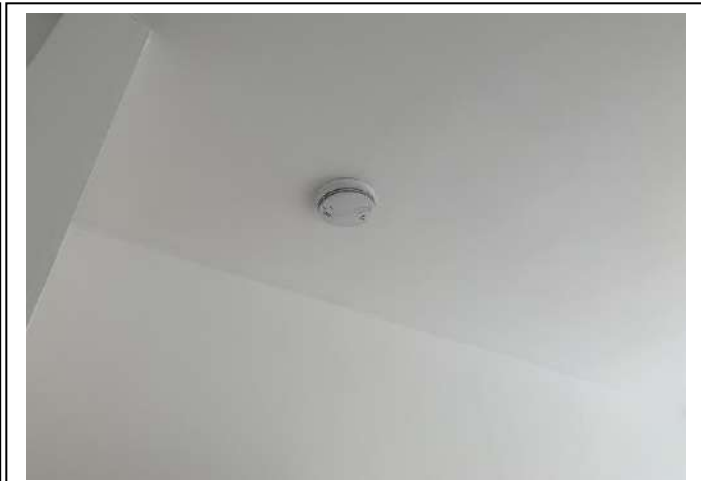
Location – Bedroom 3 Ceiling
