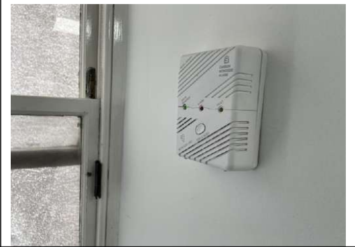
Location – Kitchen Wall
