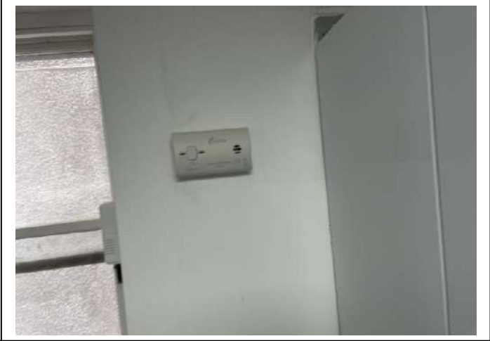
Location – Kitchen Wall
