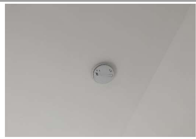
Location – Bedroom 2 Ceiling
