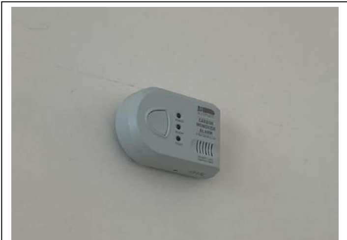
Location – Kitchen Wall
