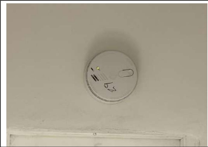
Location – Bedroom Ceiling
