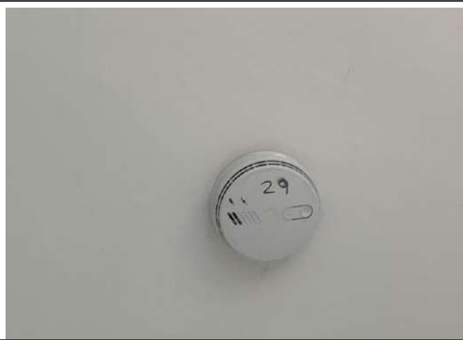
Location - Bedroom Ceiling
