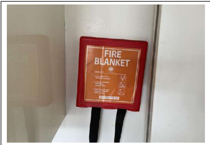
Location – Kitchen Wall
