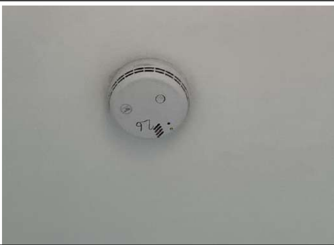
Location - Bedroom Ceiling
