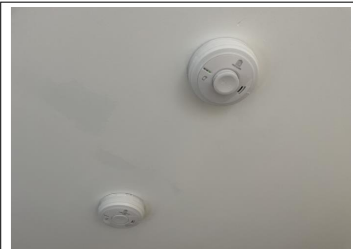
Location – Kitchen Ceiling
