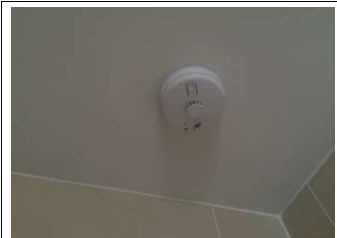
Location – Kitchen Ceiling
