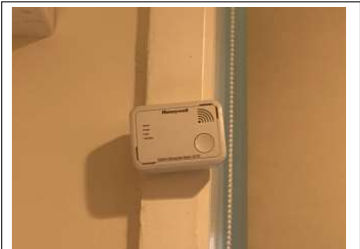
Location – Kitchen Wall
