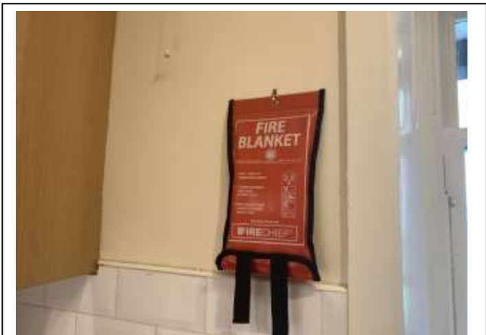
Location – Kitchen Wall
