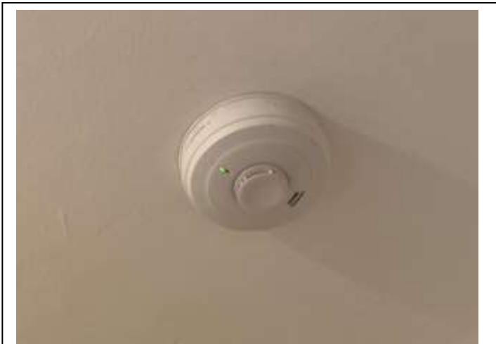
Location – Kitchen Ceiling
